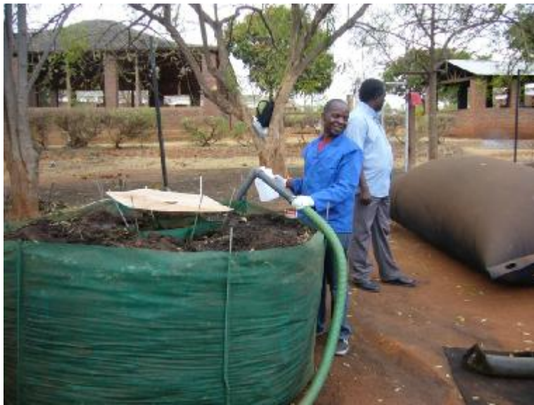
Flexigester 'Donut' for effluent disposal and gas holder full of biogas, June 2014
